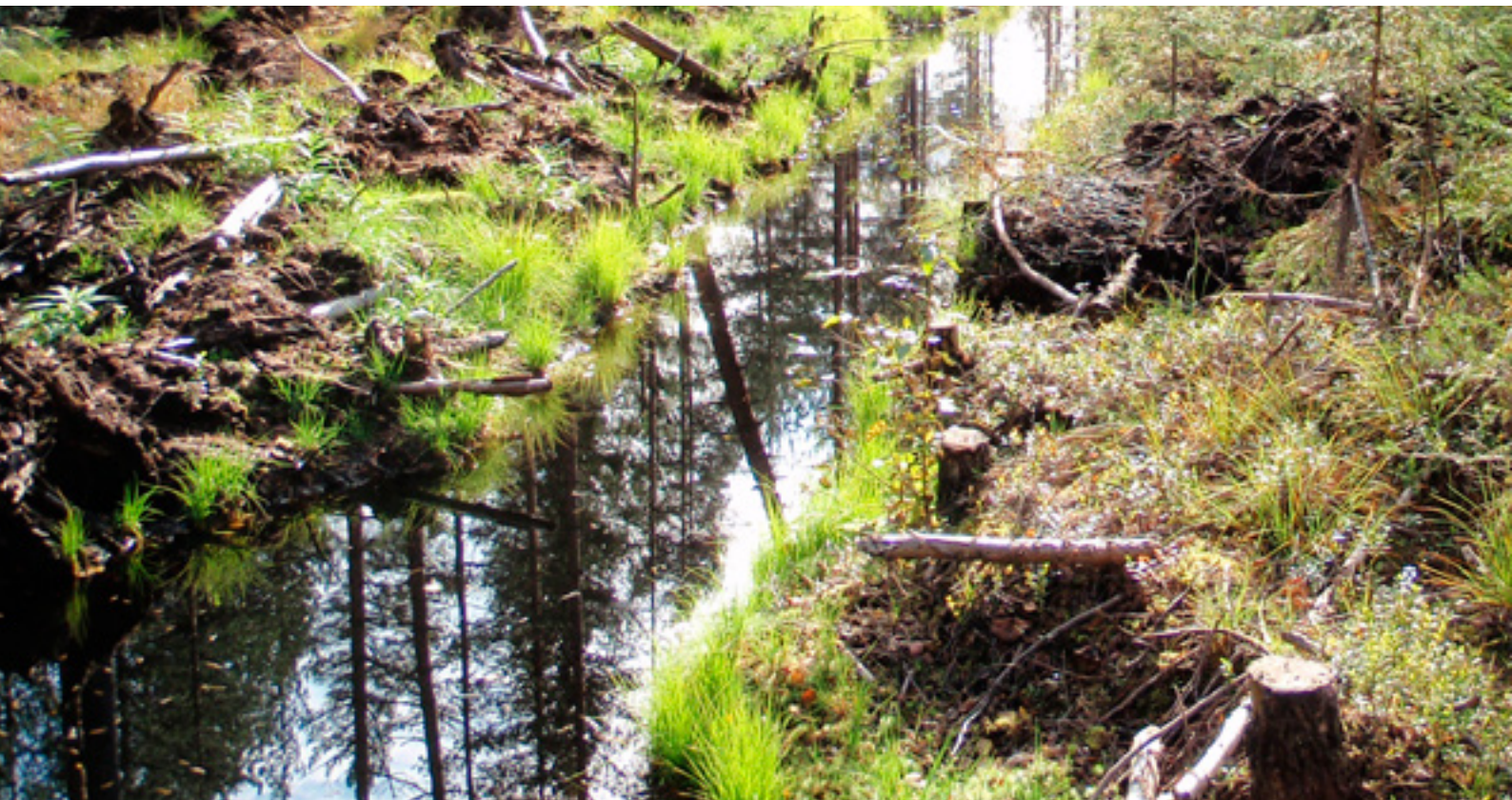
Forest drainage alters the natural water regime and productivity of a forest. FSC prohibits the drainage of previously undrained forests, although undrained forests are typically no longer drained. Photo by Henrik von Stedingk / FSC Sweden.
